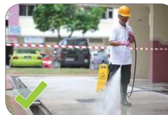
Figure 14: Spray jet (safe use)
