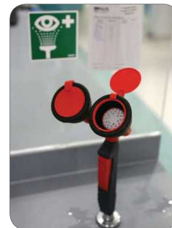
Figure 27: Emergency eyewash with flexible hose located next to a wash basin.
