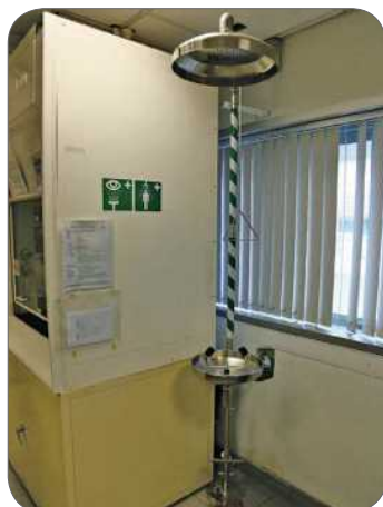
Figure 28: Safety shower with integrated eyewash and hand/ foot controls.
