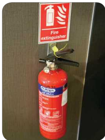
Figure 30: ABC dry chemical fire extinguisher.
